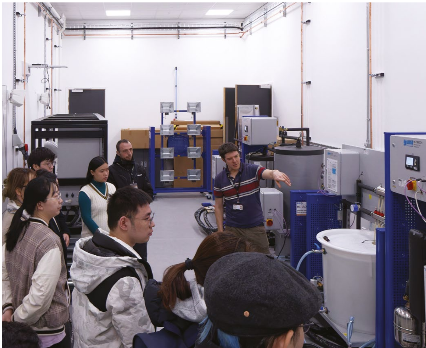
Toby Cambray demonstrates a modular heat pump system at UCL Here East (image credit: Edward Barrett)
