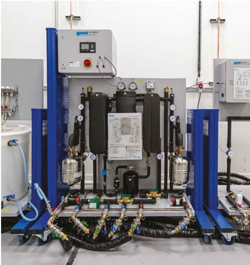
Figure 4. The modular heat pump system (HVAC Lab) (Image credit: IEDE staff)
